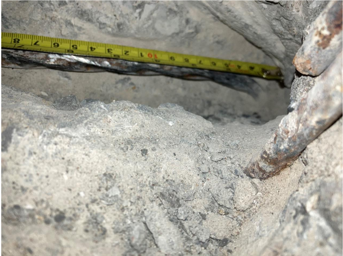
Photograph 3: External Wall Junction Curtailment of Tie
