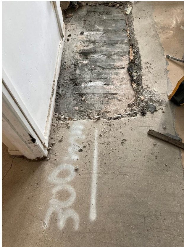
Photograph 6: Flat No. 91 Floor Crack
