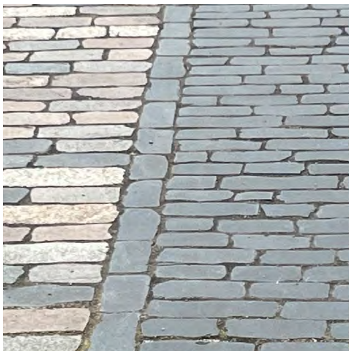
CBP2: Projects elsewhere in Bristol city centre have demonstrated that historic sett surfaces can be retained whilst significantly boosting accessibility. (Source: DK-CM)
