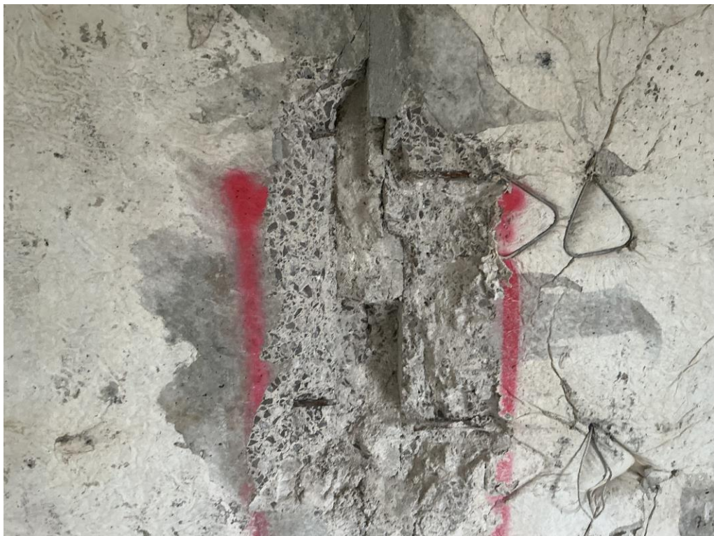
Figure 19 – Charleton House precast panel joint and exposed reinforcement with blockwork ties left in position from casting and not pulled out for use.
