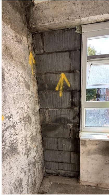
Figure 29 - Removed blockwork showing missing or unused wall tie
