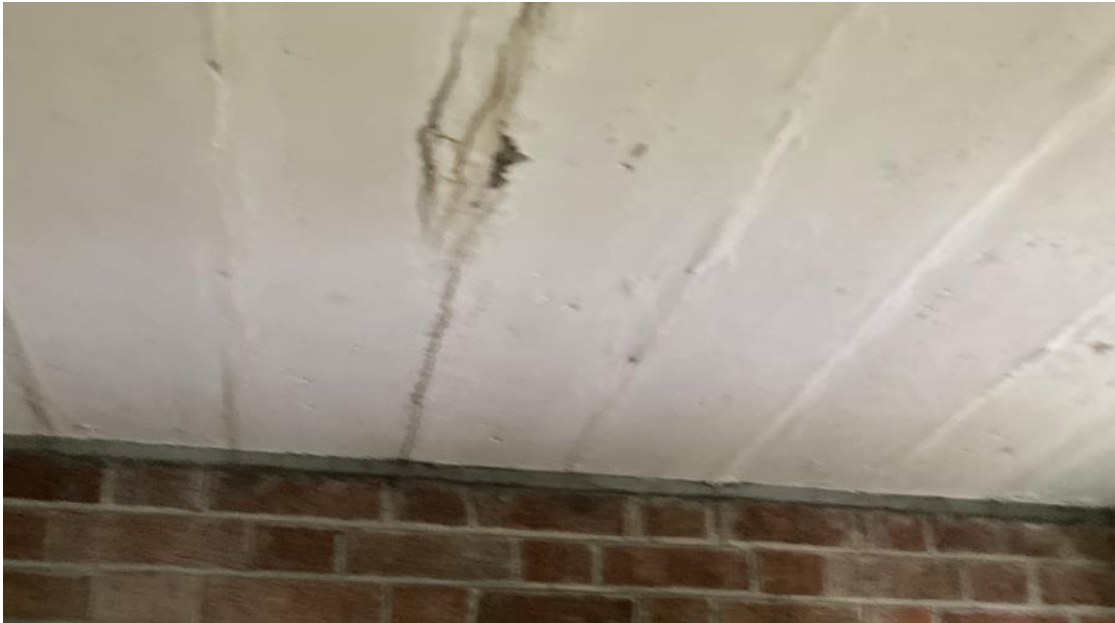
Figure 11 – Individual gothic beam floor found to be of poor quality with poor compaction widely noted.
