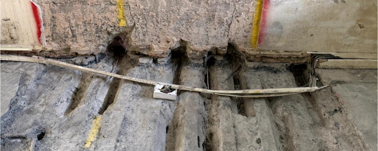
Figure 15 - Flat 20 flank wall inconsistently installed floor ties
