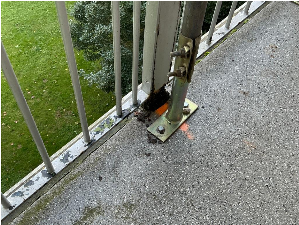
Figure 13 - Corroded balustrade connection.
