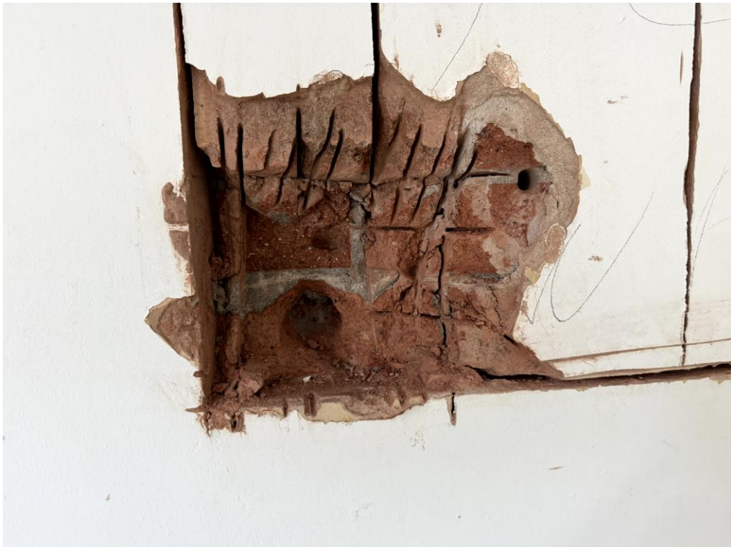
Figure 14 - Flat 14 brickwork external skin breaking out and 22mm depth check hole.
