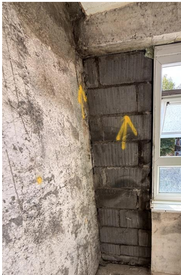
Figure 12 - No wall ties installed between blockwork and cross walls – Flat 18.
