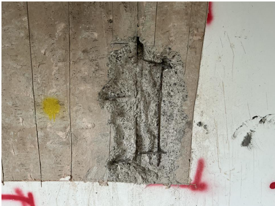
Figure 16 - Haviland House precast panel joint and exposed reinforcement
