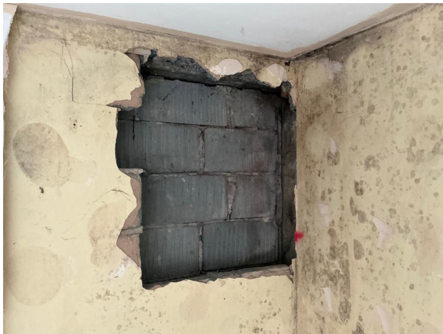
Figure 27 - Removed blockwork showing missing or unused wall ties
