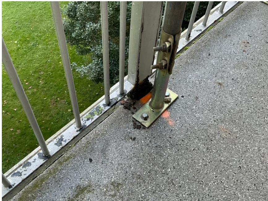
Figure 12 - Corroded balustrade connection with temporary support installed.
