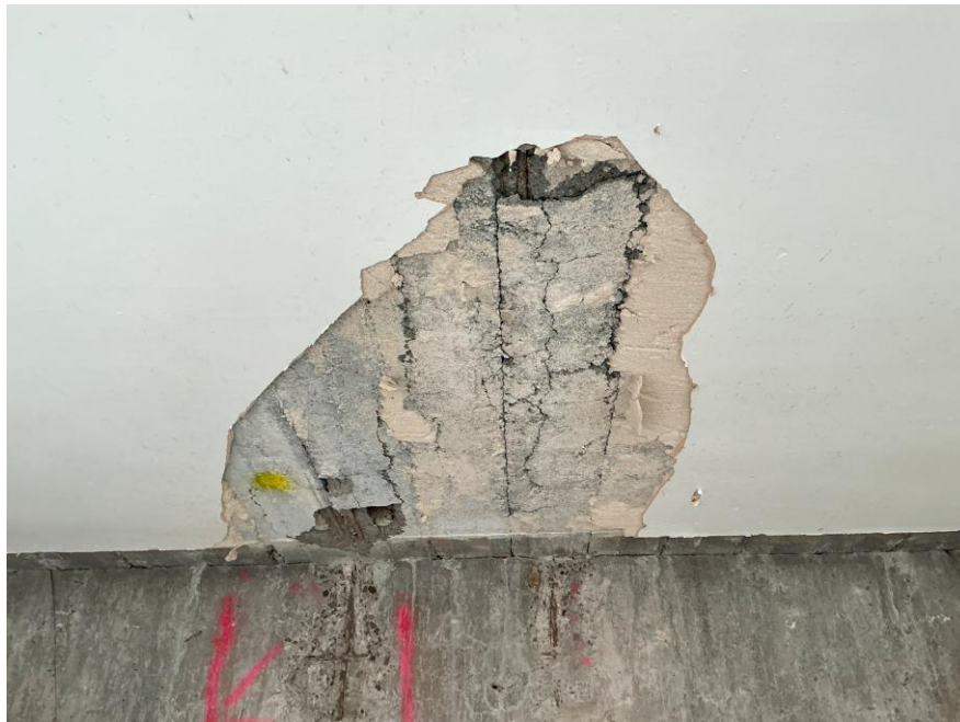
Figure 10 – Individual gothic beam floor found to be of poor quality with extensive concrete spalling.
