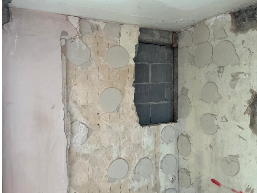
Figure 11 - No wall ties installed between blockwork and cross walls.
