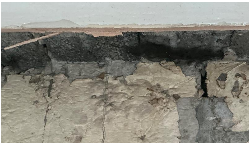
Figure 10 – Individual gothic beam floor found to be of poor quality with poor compaction widely noted.
