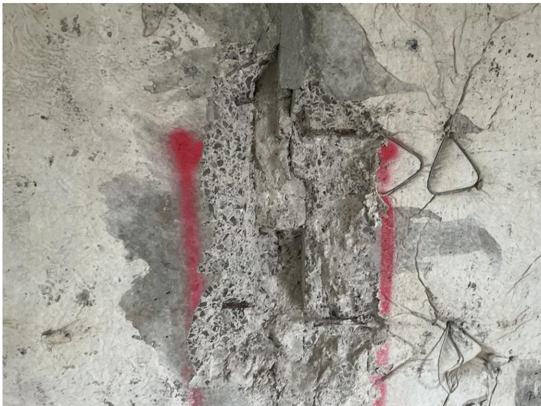
Figure 16 – John Cozens precast panel joint and exposed reinforcement with blockwork ties left in position from casting and not pulled out for use.
