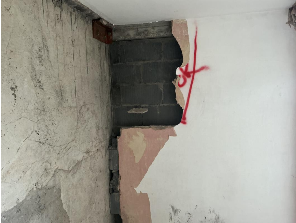
Figure 28 - Removed blockwork showing missing or unused wall tie
