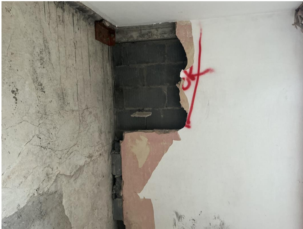
Figure 11 - No wall ties installed between blockwork and cross walls – Flat 18.
