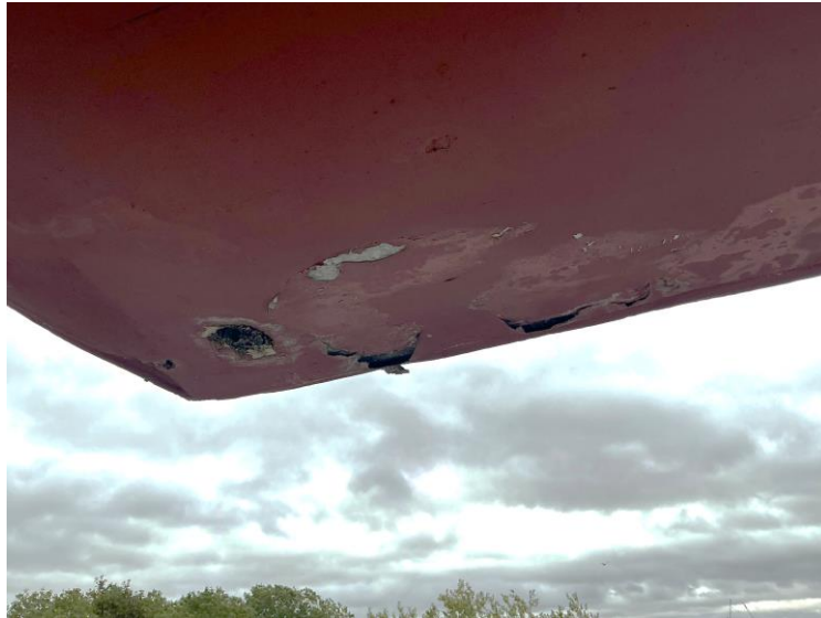
Figure 13 – Poor condition to underside of balcony
