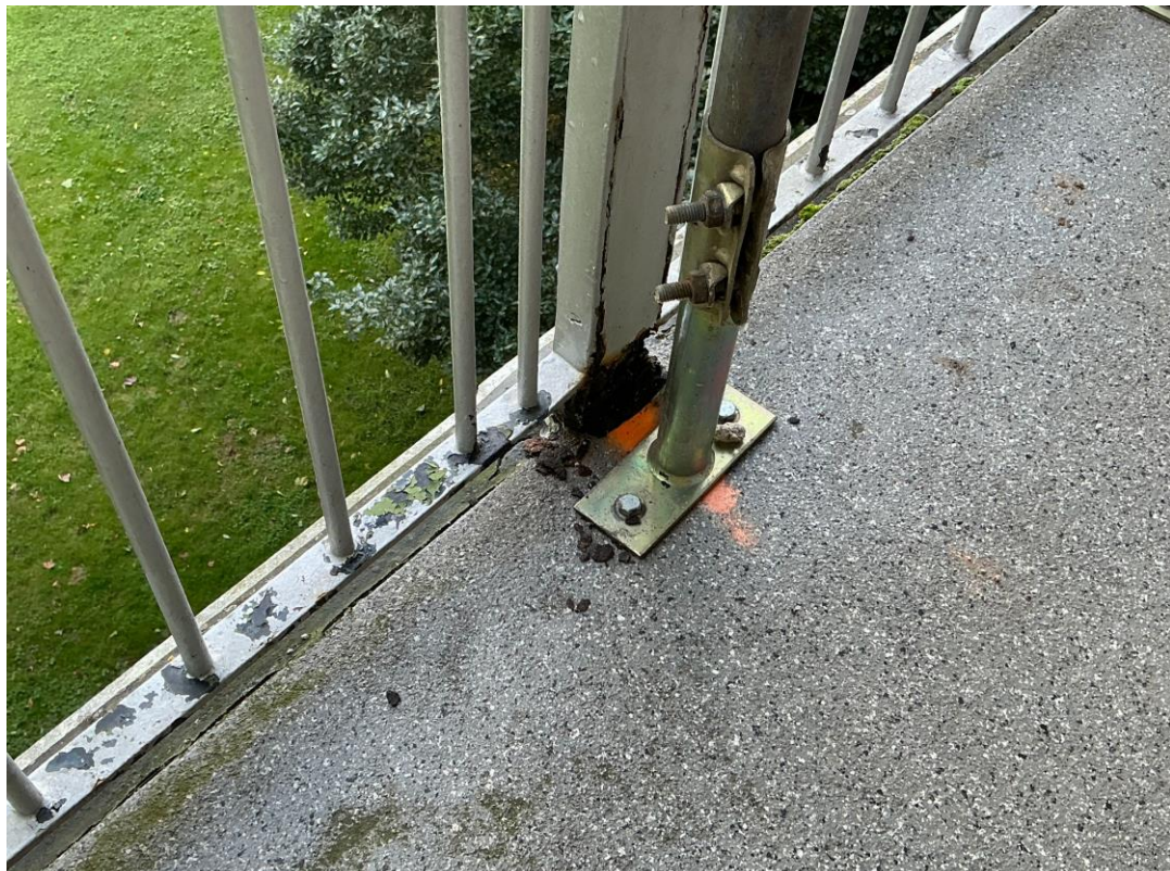
Figure 12 - Corroded balustrade connection with temporary support installed.
