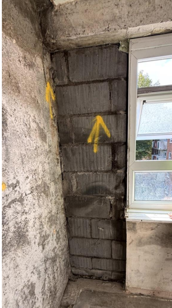
Figure 22 - Removed blockwork showing missing or unused wall tie.
