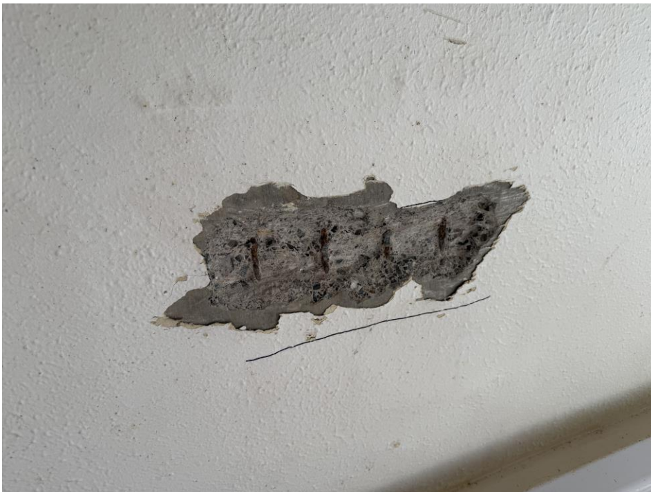
Figure 9 - Exposure of soffit reinforcement in Langton House
