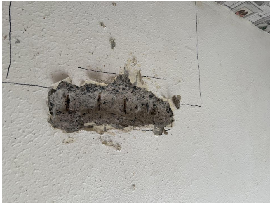
Figure 16 - Site photo of soffit break-out in Langton House
